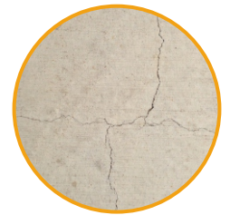
Hair Line Cracks
