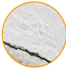
Horizontal & Vertical cracks
